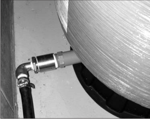
Figure 24-1: Hose from RO water outlet connected to reserve tank
