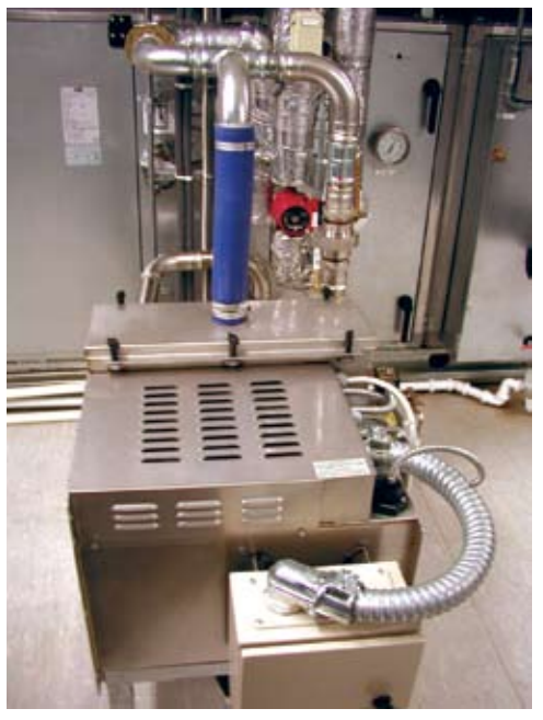
A Vaporstream Model VLC-9-1 installed in the Rikshospital, Oslo
