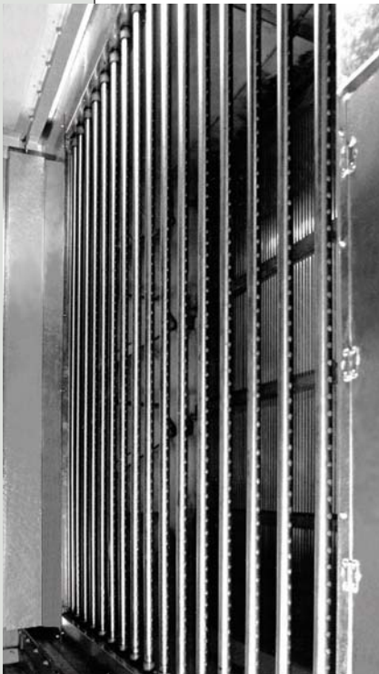
PHOTO A. Typical panel of uninsulated stainless-steel steam-dispersion tubes spanning the height and width of an AHU. The tubes discharge steam from both sides, perpendicular to airflow.
