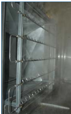
Installed in an AHU
